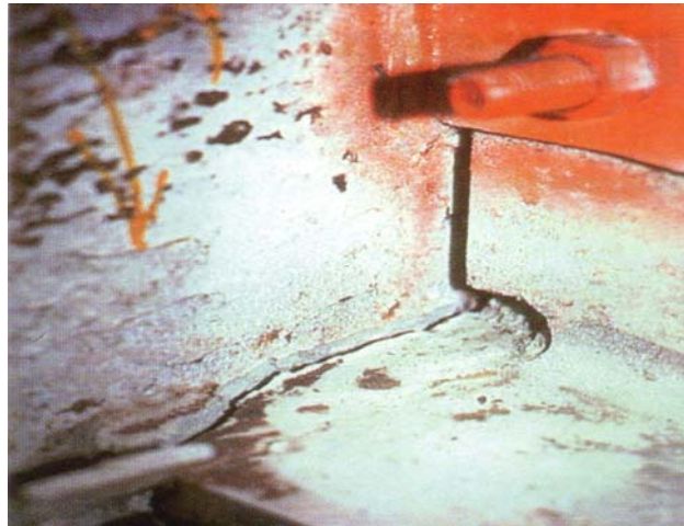
Pre-Northridge Connection - Bottom Beam Flange Weld Fracture. This Fracture Mode is a Result of Large Stress and Strain Gradients Across and Through the Beam Flanges and Welds.
