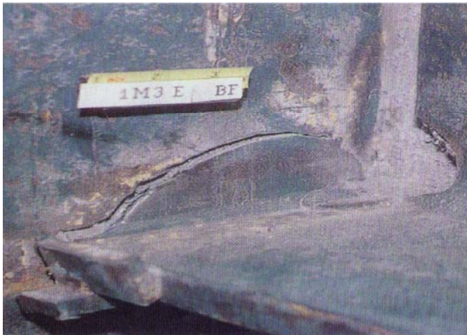
Pre-Northridge Connection Bottom Beam Flange Fracture – Column Flange Divot Pullout. This Fracture Mode is a Result of the Prying Action Due to the Shear in the Beam Flanges.
